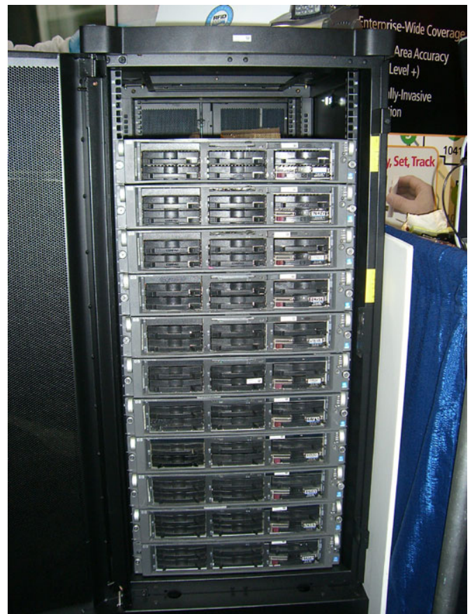
Blade servers with the Omni-ID Prox tag as you would see in a bank data center
